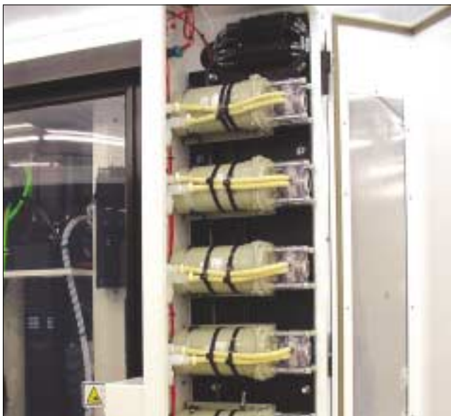
Figure 6: Photo of pumps installed on CMP tool.
