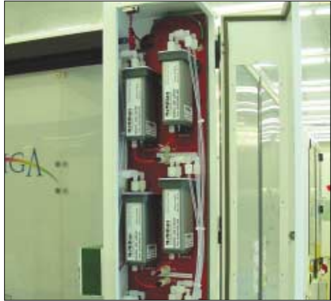
Figure 7: Photo of controllers installed on CMP tool.
